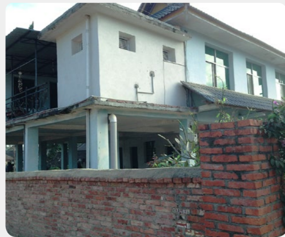
Jinghong Minsheng Rural Bank is supporting local villagers of Dai ethnic group to build houses
